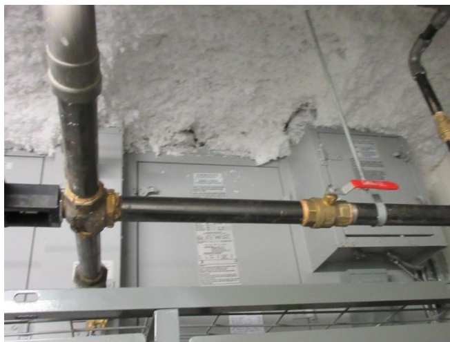
Photo 29: Typical make-up air unit.
