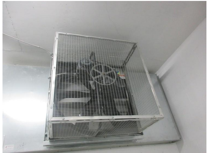
Photo 32: Typical garage exhaust fan.
