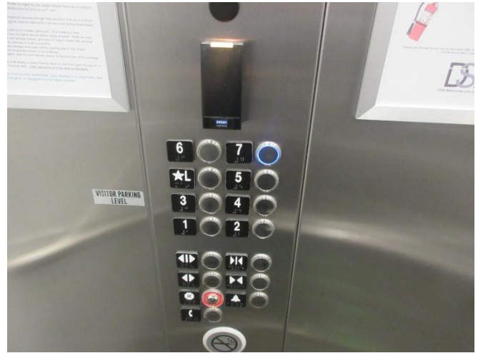
Photo 41: Typical elevator button panel.
