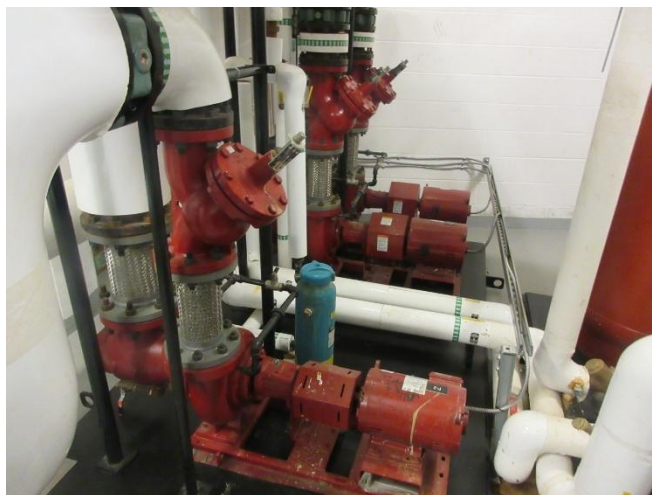
Photo 33: Heat pump and cooling loops circulation pumps.
