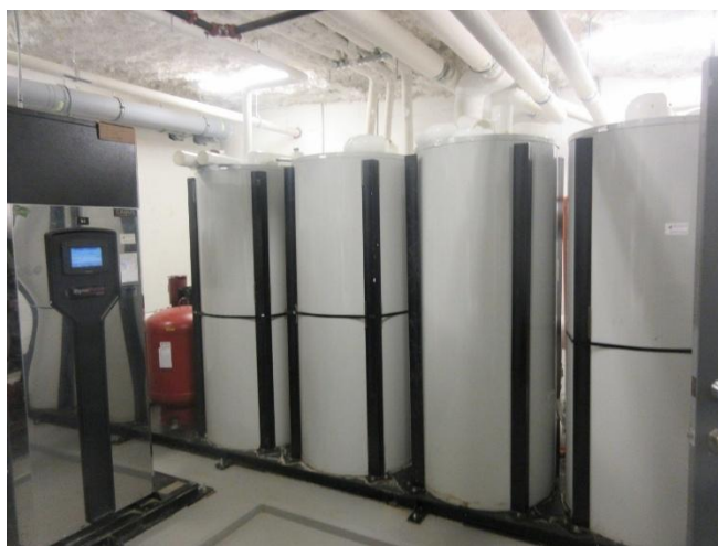
Photo 35: Hot water storage tanks.
