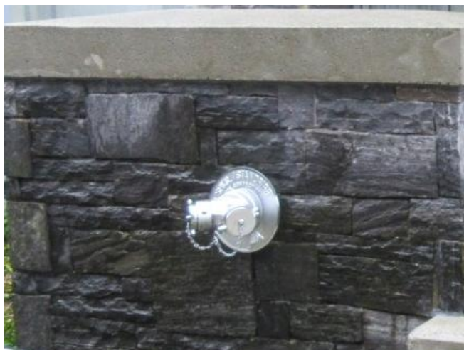
Photo 18: Typical fire department connections.
