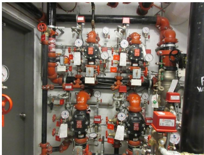
Photo 17: Fire suppression equipment.
