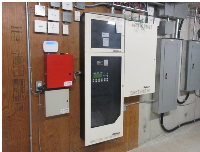
Photo 15: Typical fire alarm control and booster panels.
