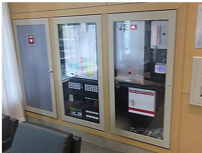
Photo 16: Typical remote annunciator panel.
