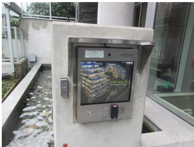
Photo 43: Typical enterphone panel and fob access reader.
