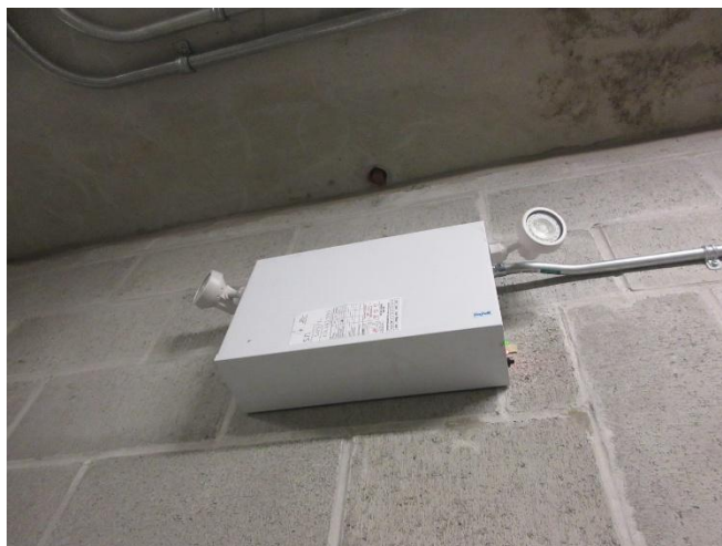
Photo 20: Typical emergency lighting unit.
