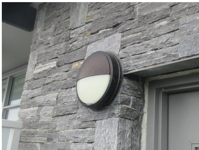
Photo 40: Typical exterior wall-mounted light.
