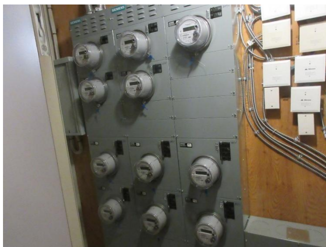
Photo 39: Typical suite meters.
