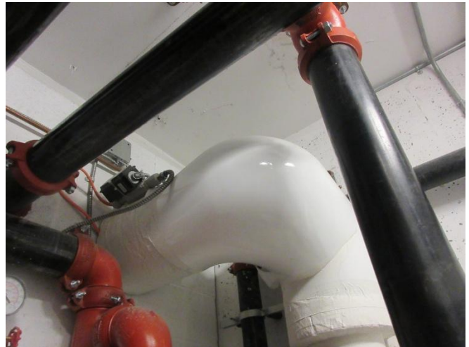
Photo 36: Combined incoming service.
