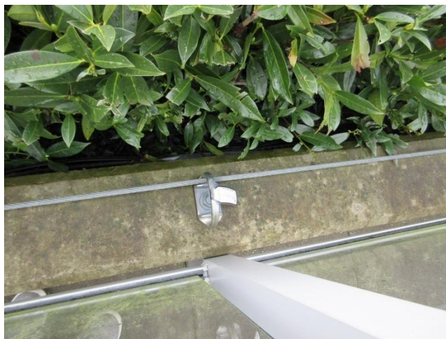
Photo 5: Typical anchor and horizontal lifeline.
