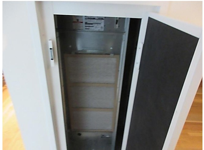
Photo 30: Typical in-suite/unit heat pump unit.
