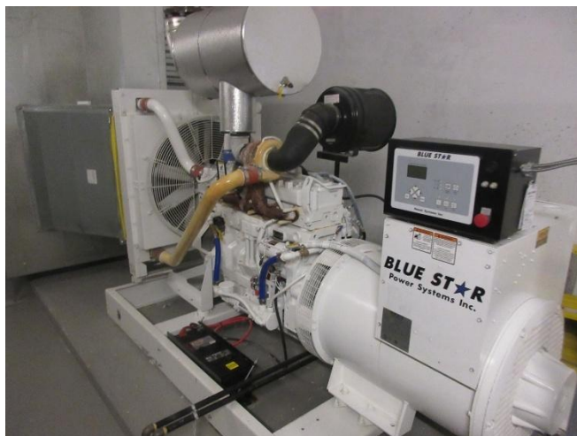
Photo 19: Emergency power generator.
