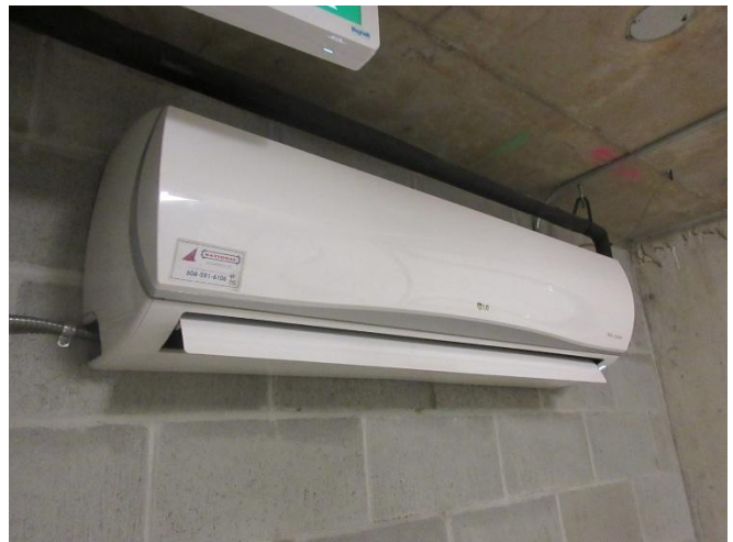
Photo 31: Air conditioning unit in electrical room.
